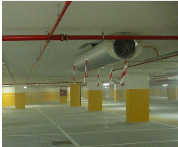
Figure 2: Car park overview with a jet fan suspended under the ceiling.
